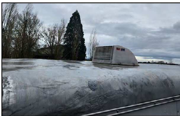
Trailer roof, before and after Jack repaired the damage caused by a tree that fell in a wind storm.
